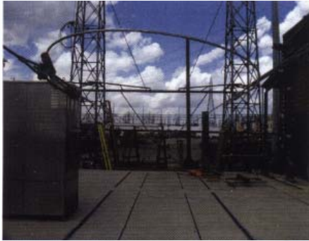
Typical Set-up for Short Circuit Test in High Current Yard
